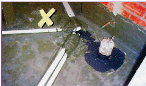
Poor arrangement of pipes
