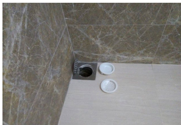
Joint at floor trap covered with grout
