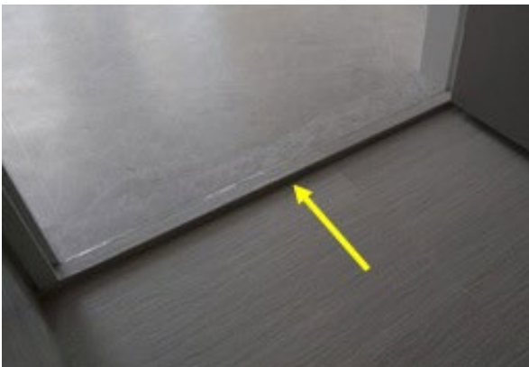
Threshold to reduce water ingress
