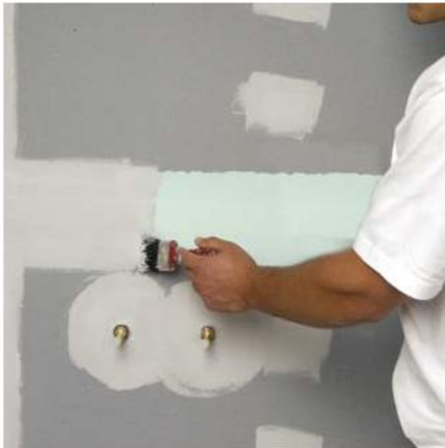
7. Apply two liberal coats of Wet Area SealCote at all joints, junctions, penetrations and fastener heads.
