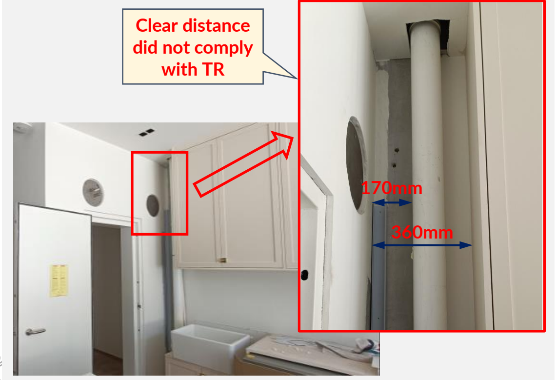
Example of non-compliance
