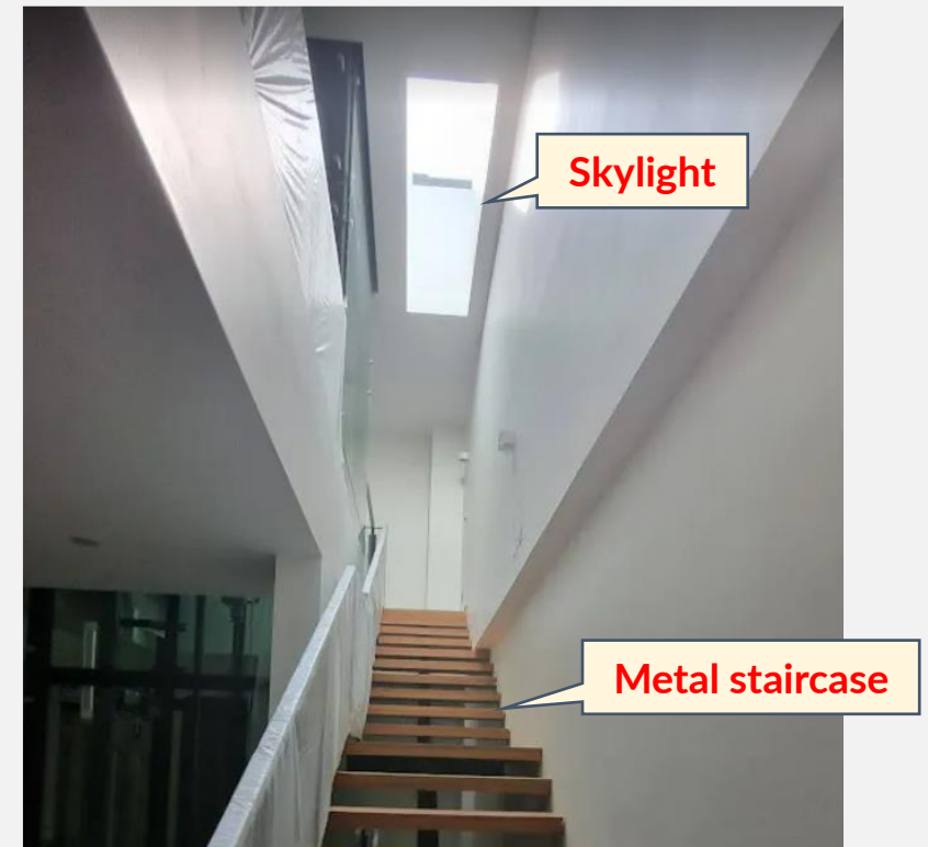
Example of non-compliance
