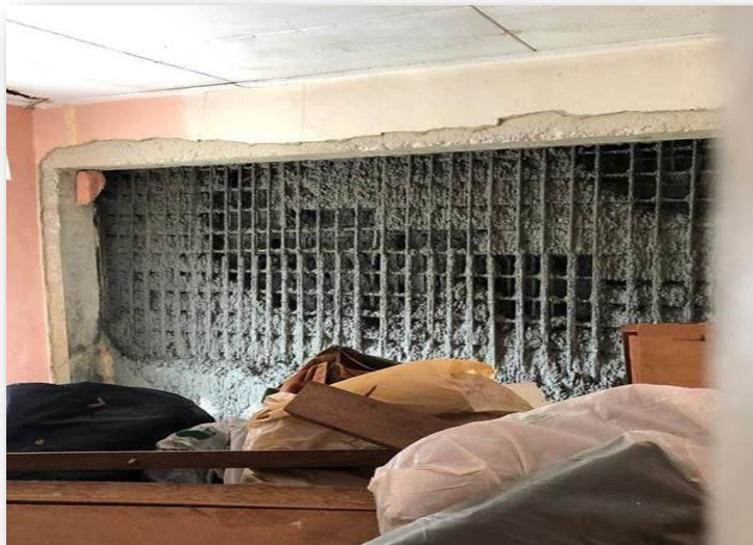
Example of partywall collapse during casting of new RC wall abutting it
