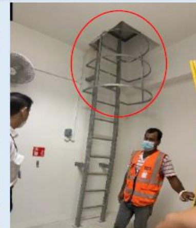
Figure H—VIII: Locked-entry cat ladder / hatch doors; with signage to indicate maintenance area
