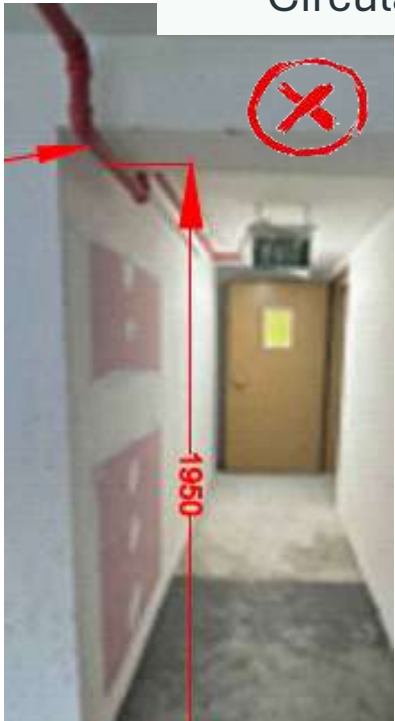
Sprinkler running <2.0m
