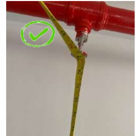
2m clearance from underside of sprinkler head
