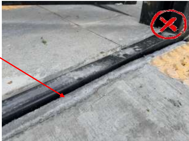
Accessible route doorway not leveled
