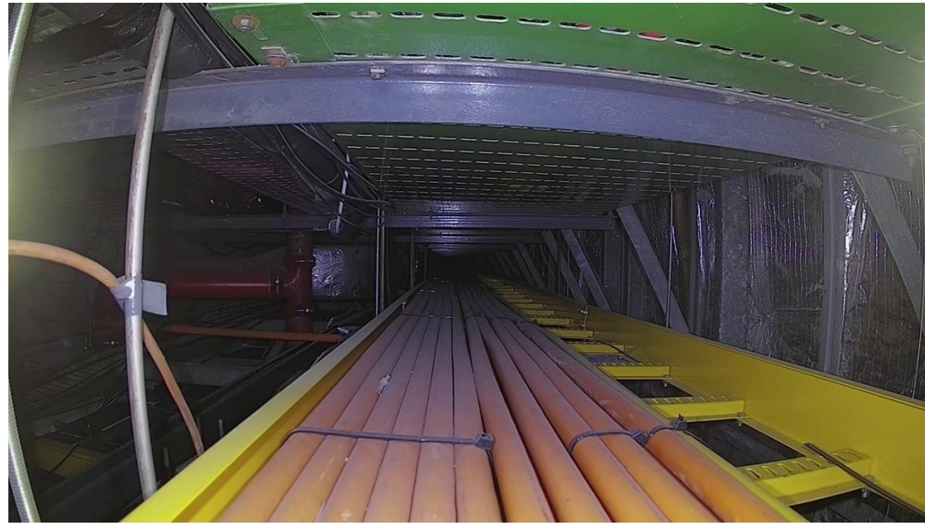
Cable Trays, MEP Infrastructure
