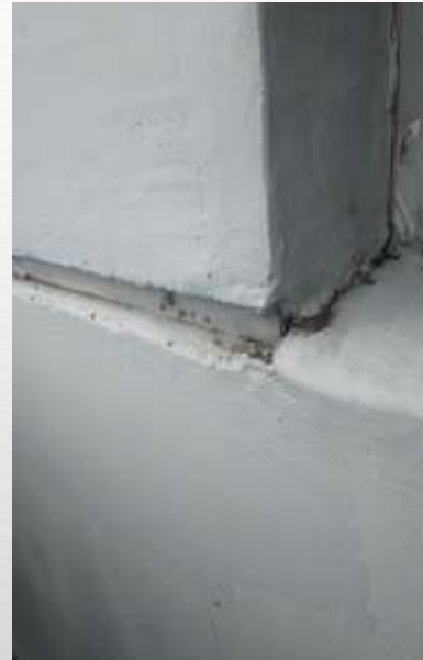
Poor joint details.
