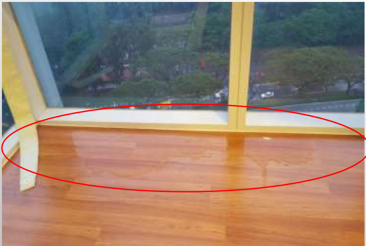
Water seep through grouting.
