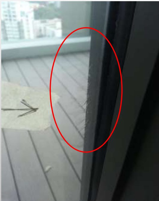
De-lamination observed on edge of glass.
