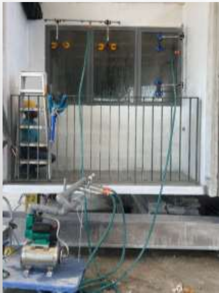
Conducting field water test in 501.2 method of test.
