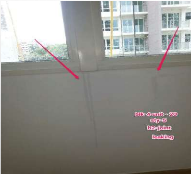
Sign of water seepage through the bottom sill and mullion during site field water test.
