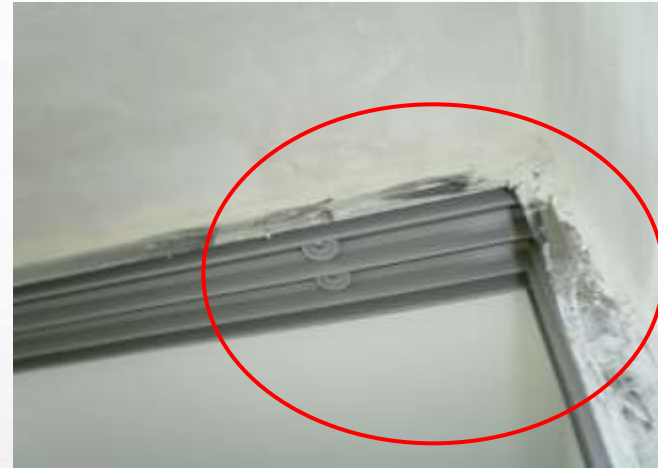
No protection during wall painting.
