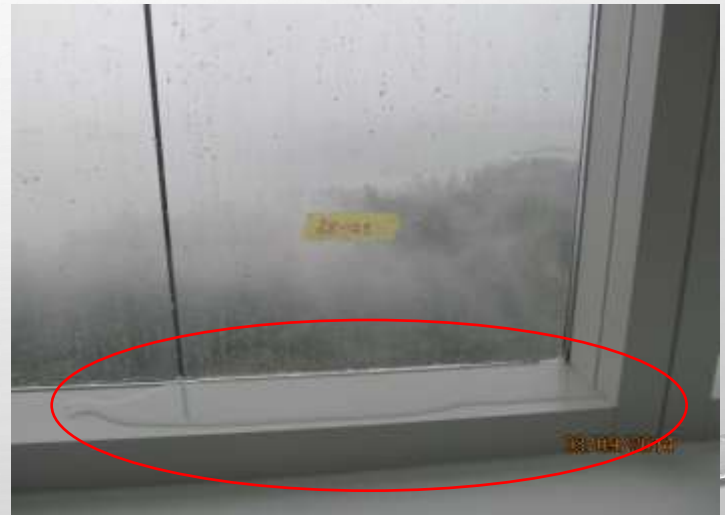
Water seep through poor corner joints.
