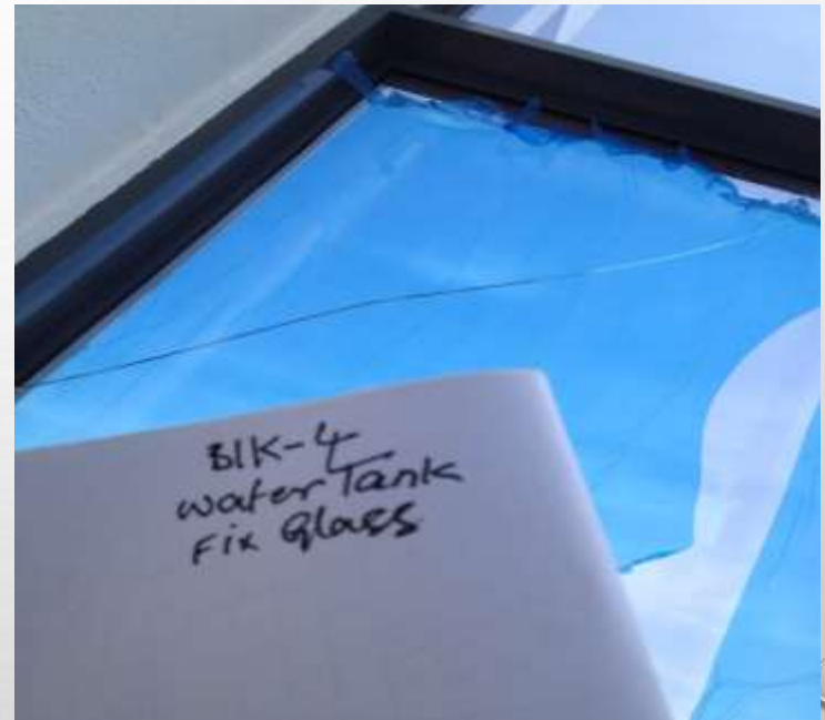
Glass broken by cleaning contractor.
