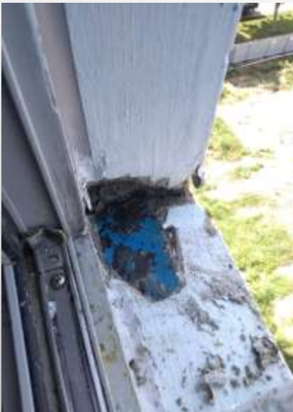
Poor treatment between alum frame and plastering.
