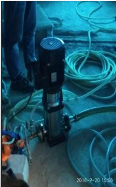
Electric pump – Filter from water tank
