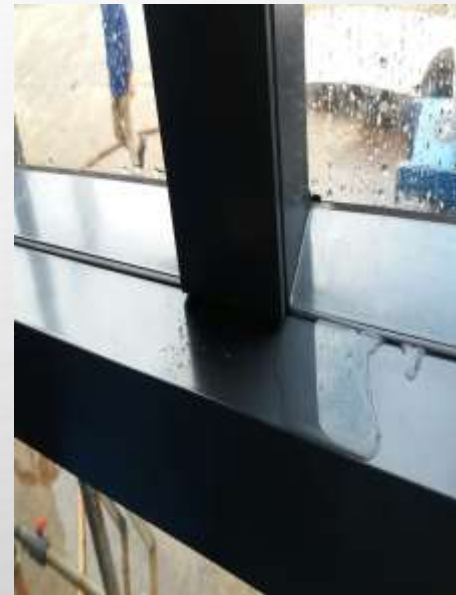
Water seepage is observed to overflow from the sash / transom.
