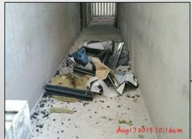
Fallen window frame
