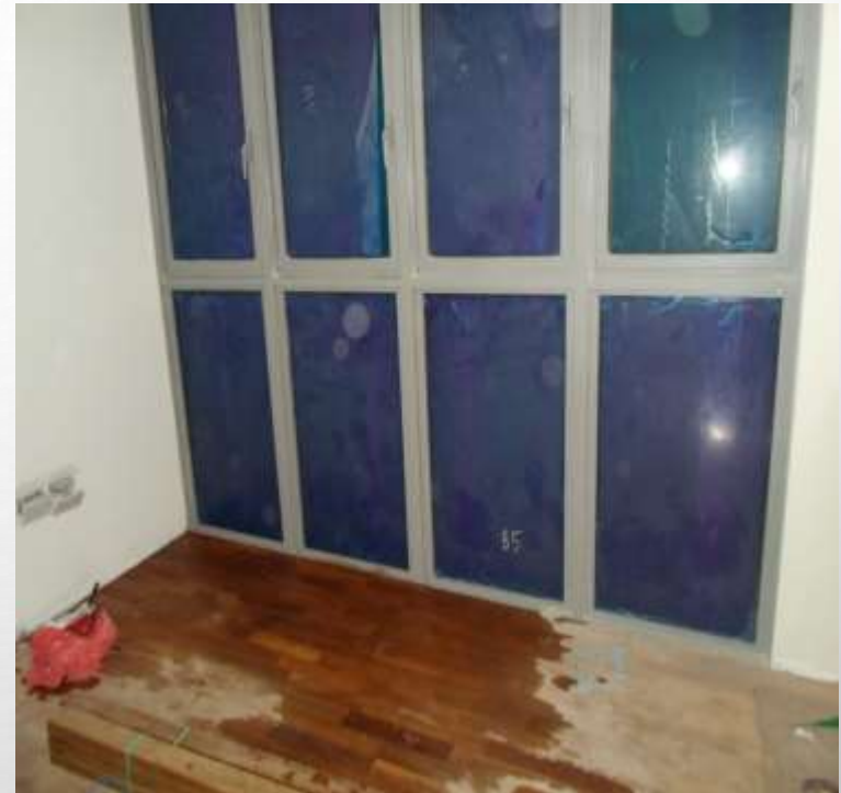
Major seepage through full height window during field water test.
