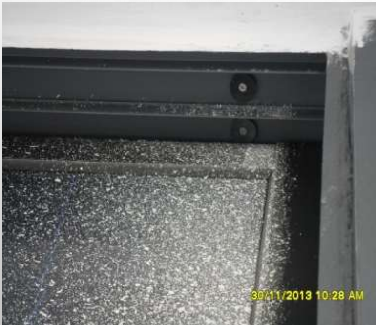
No protection during spray texture coating on external wall.
