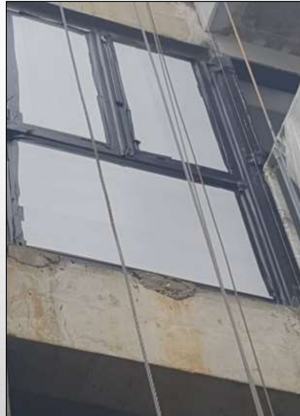
Poor infill of grout on kerb – result in water seepage.
