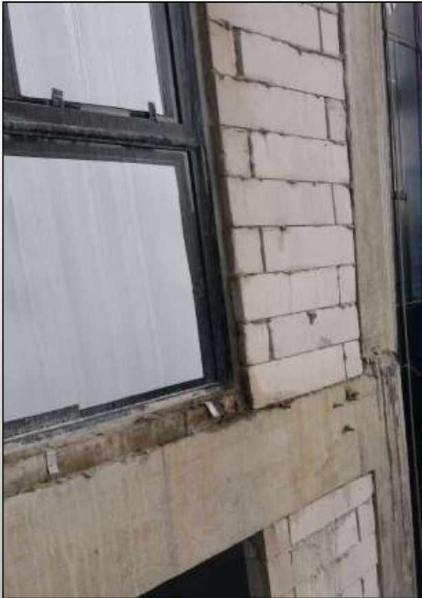
Water seepage through hollow block joints.
